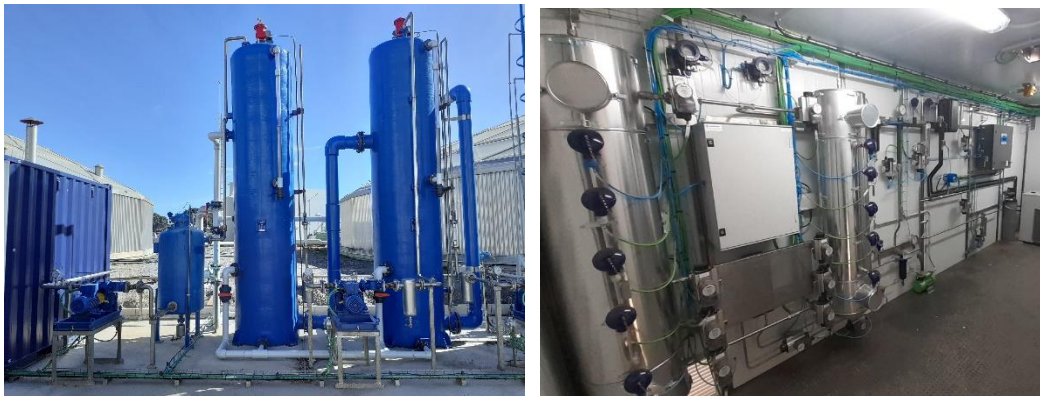
Figure 8. ABAD Bioenergy up-grading columns (left) and polishing container inside view (right)
