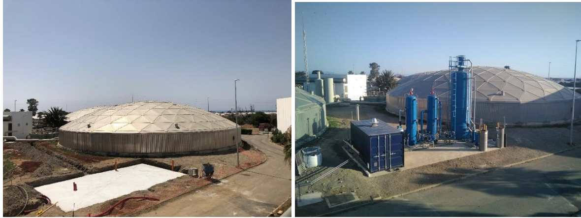
Figure 7. Area 1 view: concrete slab during civil works (left) and ABAD and PUSH plants (right)
