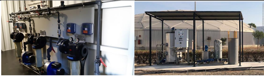
Figure 10. Struvite plant (left) and hydrolysis plant installed at its final location (right)
