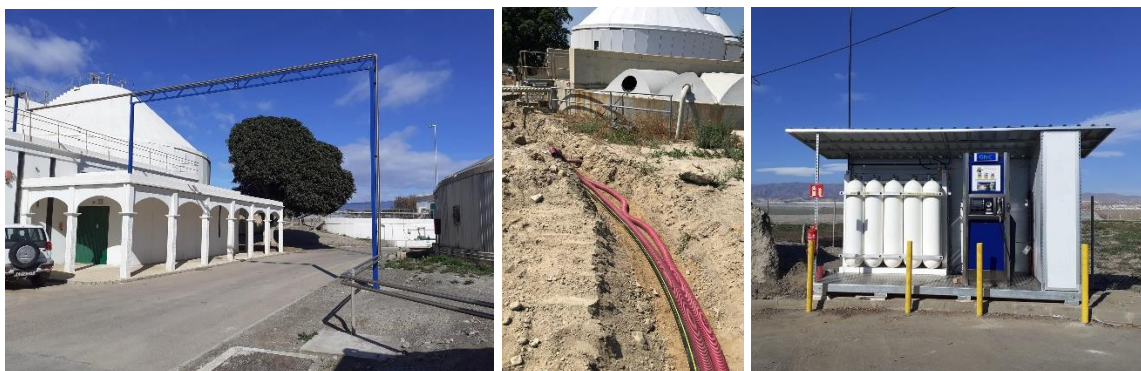
Figure 9. biogas aerial pipes (left), biomethane underground pipe (centre), refuelling station (right)
